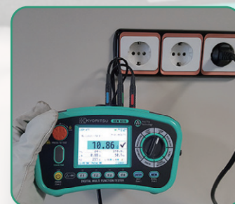
Loop test from a wall socket
